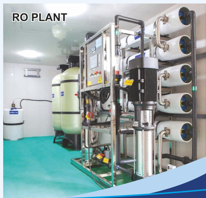
STP & ETP PLANT
